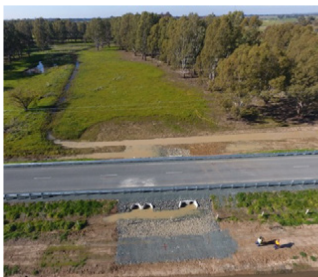
Figure 6: Hybrid-DCD drainage with installation of road culverts to remove obstructions and open up the flow path along a natural drainage line.
